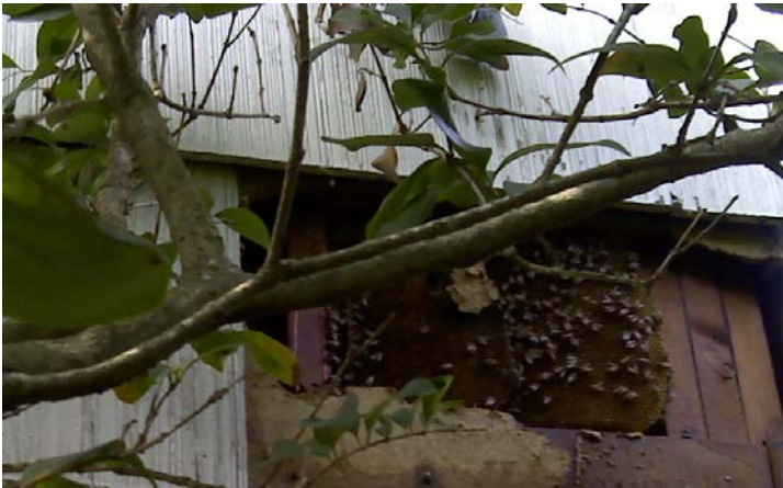
Exterior wall of a two-story residence on Midlane opened to expose and remove beehive built between floors
